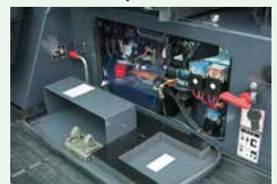
•Generator •Starter motor
